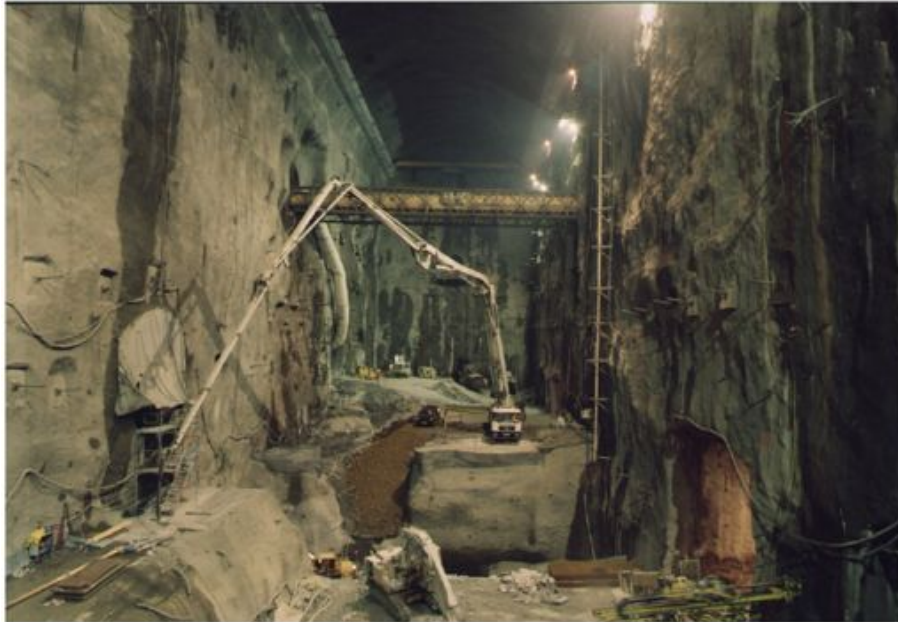
Figure 75: The construction of the Robert Bourassa hydropower station in Quebec, Canada. Drill and blast was used to excavate the powerhouse with dimensions 296 m by 25 m by 47 m. More than 11,000 rock bolts were used.
