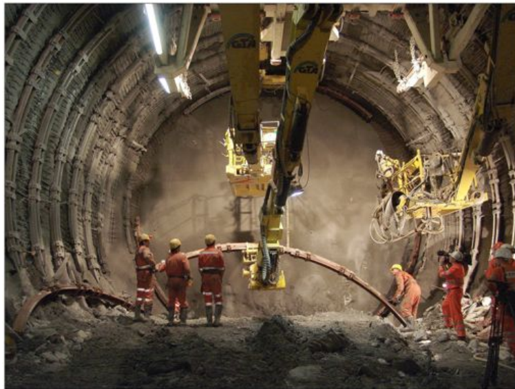
Figure 81: Support of the tunnel walls can be erected in parallel to the drilling process.
