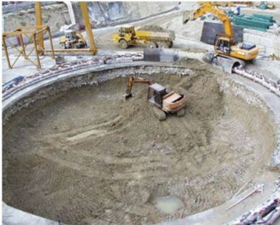
Figure 86: The construction of the CMS access shaft for the LHC project at CERN, Geneva. This shaft has an 18 m diameter and the entire CMS experiment was lowered through it. To facility its construction, the ground at the shaft walls was frozen.
