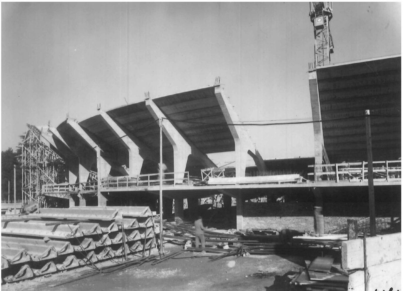
Fig. 6. The construction site: on the ground the prefabricated elements of the steps.
