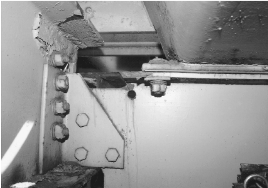
FIGURE 2-18 Fatigue cracks at the floor beam of Throgg's Neck Bridge in New York (W. Chen and L. Duan, 2000)
