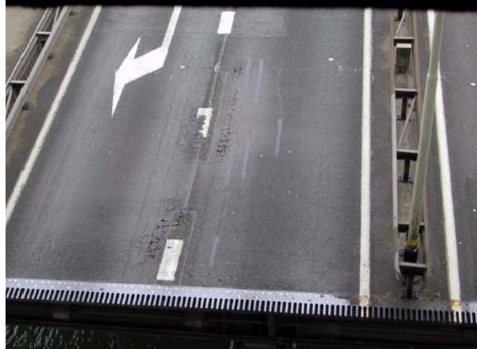
FIGURE 2-19 Visual observations indicating deck plate cracking fixed bridge (Dong et al., 2004)
