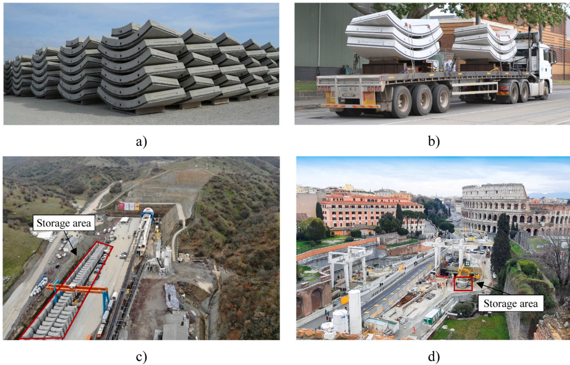
Fig. 2. Storage and transport of the precast segments. a) Storage; b) Transport; c) Tunnel construction in rural areas (image from the website: www.sabah.com ); and d) Tunnel construction in urban areas.
