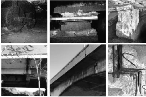
Figure 7. Detail of deterioration in supporting device and reinforced concrete half-joint (courtesy of Rome Municipal Archive, Bridge Office and Micheloni et al. 2018).
