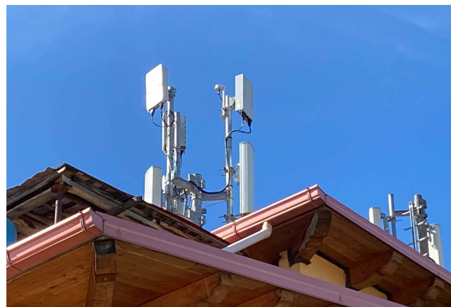
FIGURE 2. Roof-top FR2 gNB.
