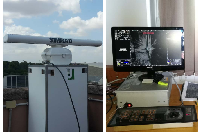
Fig. 2. Radar body on moving platform (left) and console with PPI (right).
