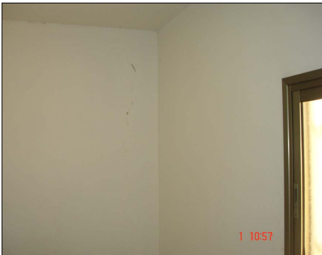
Photo 13:- Cracks through the walls of a house in Bani Naim area as a result of neighboring quarrying land vibration.
